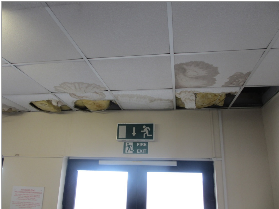
Figure 2: Evidence of water entering terminal building
